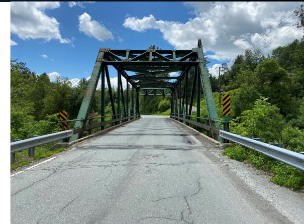
Narrow Bridge: Pedestrian, Bicycle and Snowmobile conflict
